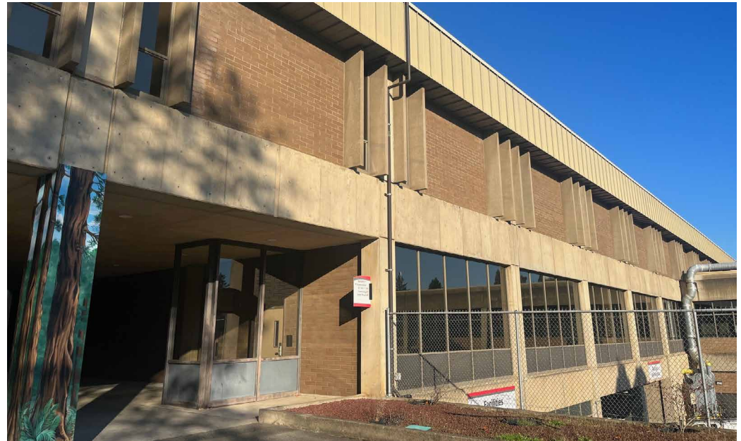
EXISTING NON-THERMAL WINDOWS EXPOSED TO EAST WIND
